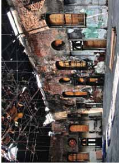
above: A view of the fire-damaged interior of Eastem Market. Courtesy of Quinn Stone Architects.
