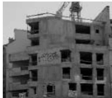
above / Typical concrete bearing wall buildings under construction in France in the 1990s. Notice the relatively small, distinct openings corresponding exactly to the locations of windows and doors.
