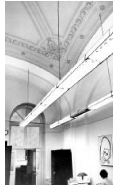
top / Photograph showing the condition of a space on the fourth floor of the Pension Building before renovation. From a thesis project for a new museum of architecture in the Pension Building, by B. Christopher Bene, University of Virginia, 1975.
